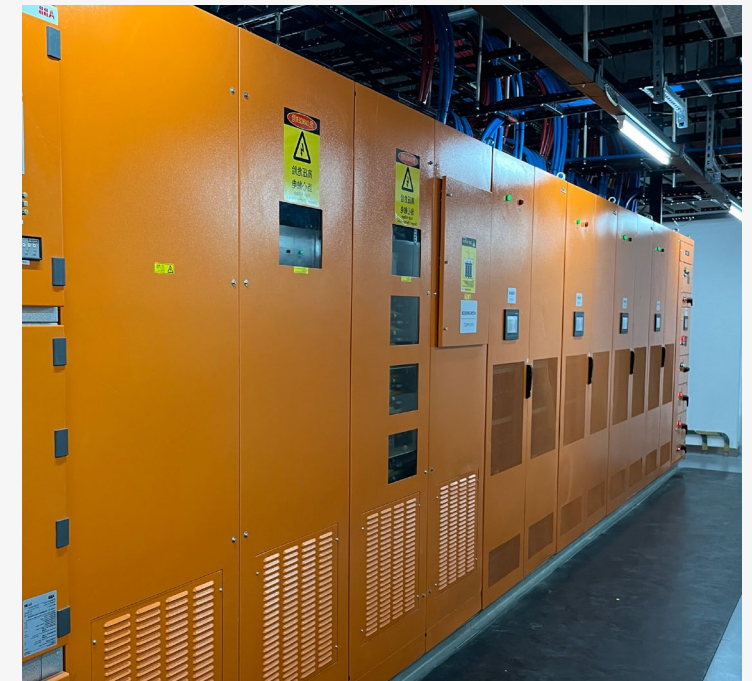
Panama power solution
